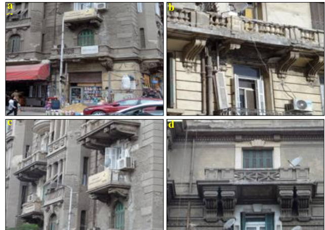
Figure (3) the various facades of the building 17 Mohamed Mahmoud St.; a. the shape of the stucco consoles and the black calcification layers on them resulting from the accumulation of aerosols from transport vehicles sample (S3), b. the loss of some parts of the stucco consoles under the balcony sample (S4), c. the different types of consoles in the same building, d. damage aspects in the form of blacking calcification on the stucco decorations.
