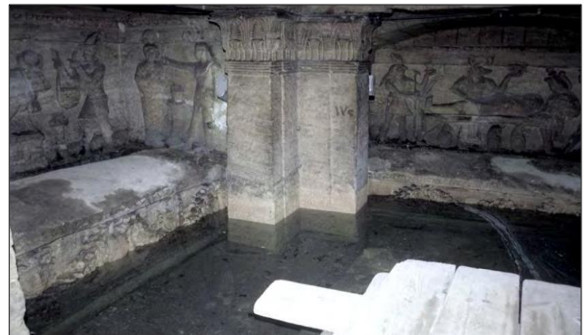
Figure (7) chamber G in the main catacombs with the high-water level (After: ARCE, 1995 )
