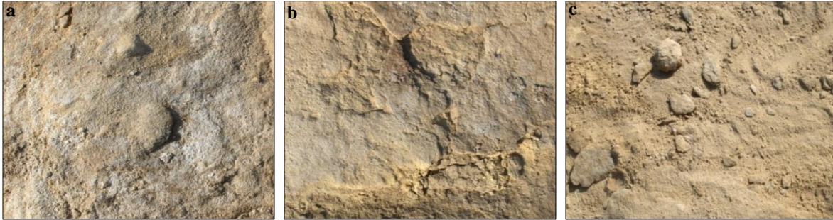
Figure (4) Shows the development stages of the stone bleeding; a. crust created, b. granular disintegration, c. stone bleeding.
