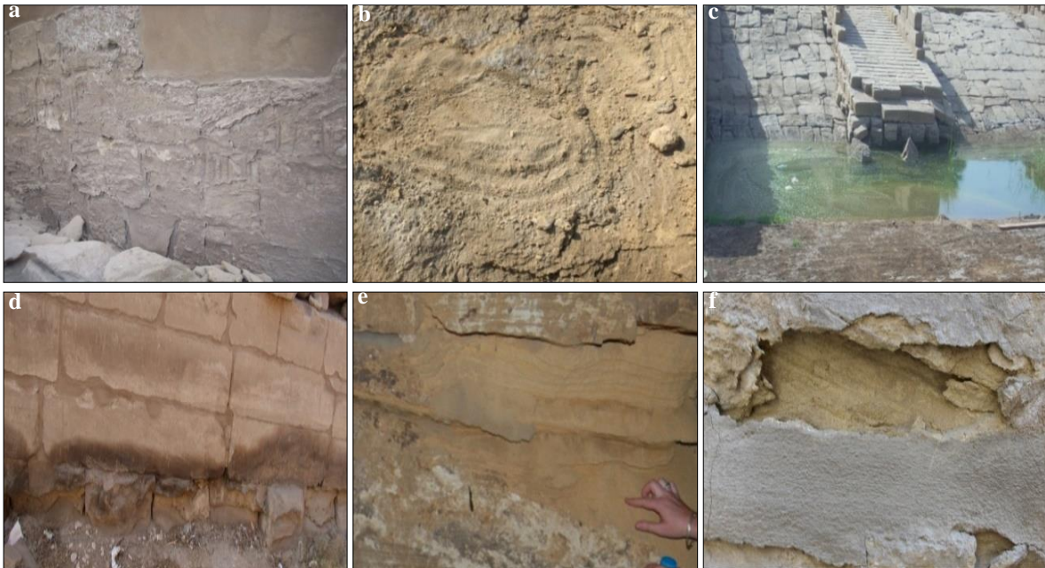
Figure (2) Shows some occurring reasons of stone bleeding affected the study areas a. depth of preparation layer of incoherent construction materials, b. salt efflorescence in some doorsteps, c. groundwater in the wall of the port below the entrance of Karnak temples, d. humidity and its effect on the Taharqa temple, f. improper restoration using black cement in the southern part of Hall two of the Holy of Holies, Temple of Ramesses III, Karnak.
