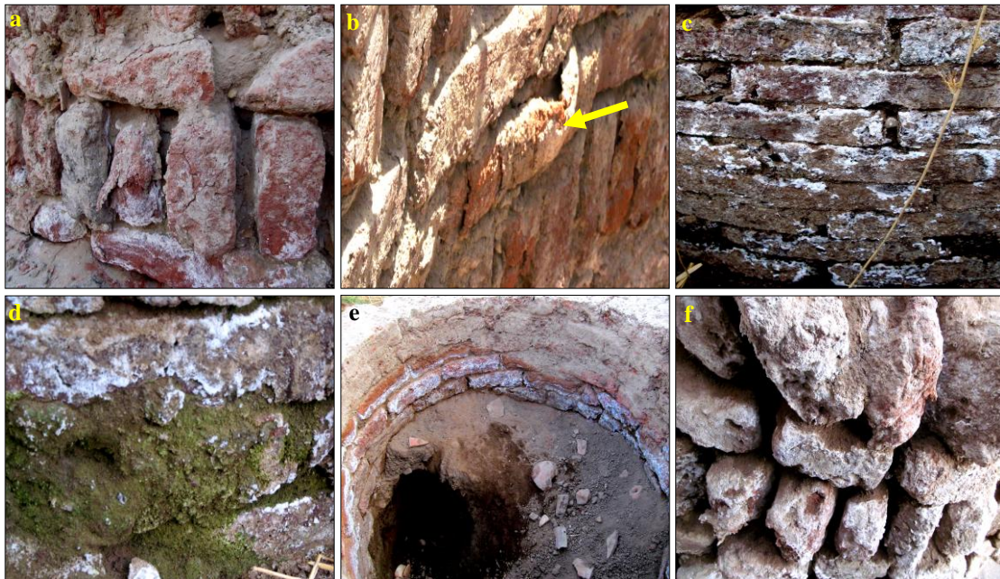
Figure (2) Shows deterioration features of water wells at Karnak temple a. exfoliation, b. crumbling, c. efflorescence, d. algae colonies, e. filling up with debris, f. partial collapse of the structure.
